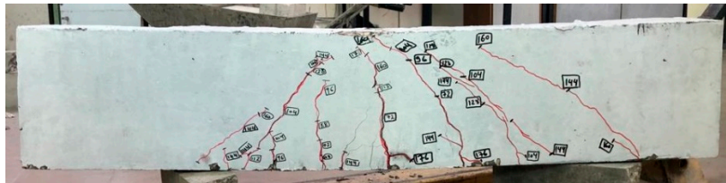
Figure 18. Crack pattern for beam PS-0.
