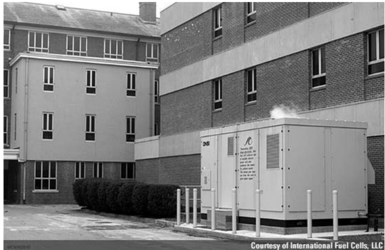
Fig. 20.10 Photograph of PC25 fuel cell unit at South County Hospital, Wakefield, RI, USA. (Courtesy of International Fuel Cells Inc.)
